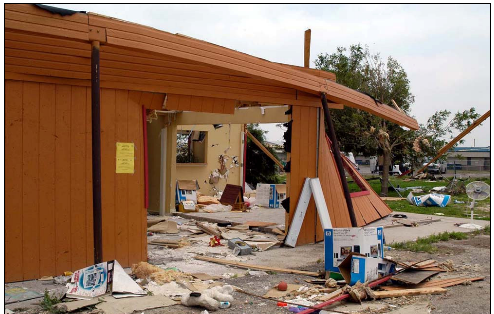
This building was severely damaged during an April 2007 tornado in Rosita Valley, Texas. (Photo by Ilan Kelman; http://www.ilankelman.org )
