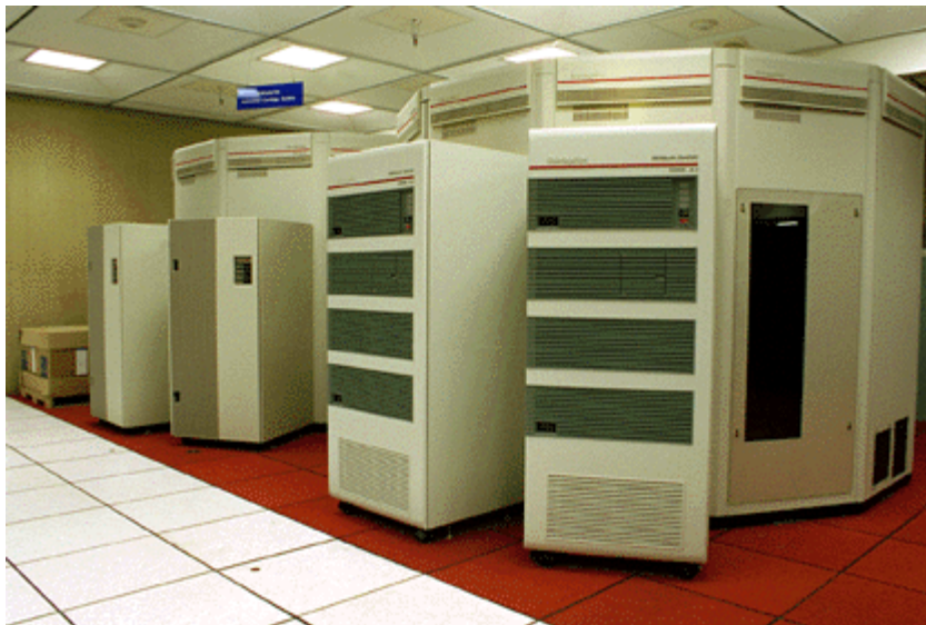
Silos old (left) and new (right) sit side by side in the SCD machine room.
