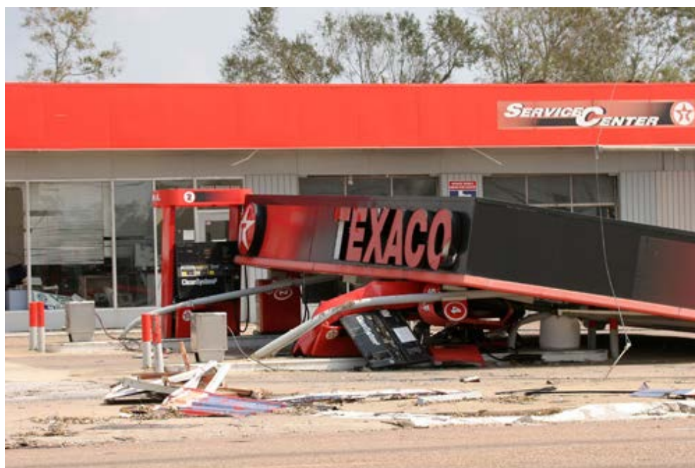
Winds from Hurricane Rita damaged structures along much of the Texas and Louisiana coasts, including this gas station in Port Arthur, Texas. (Photo by Bob McMillan, FEMA.)
